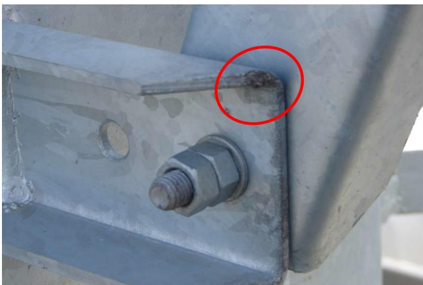
Fig. 3. Appearance of corrosion in the form of oxidation on a profile edge (marked in red).
