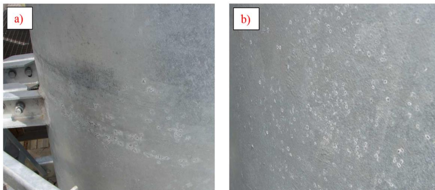
Fig. 7. 'White rust' on the surface of zinc coating.
