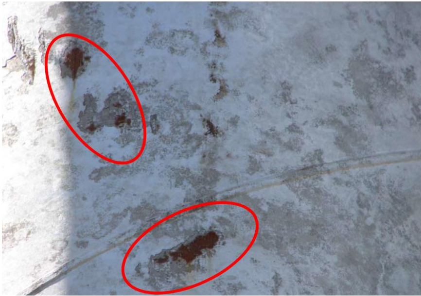
Fig. 2. Surface oxidation of the material under the coating as a result of zinc coating flaking off (marked in red).
