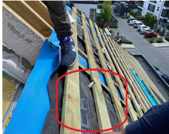
Fig. 3b. Timber battens for a coated steel roof panel (marked in red) [7].
