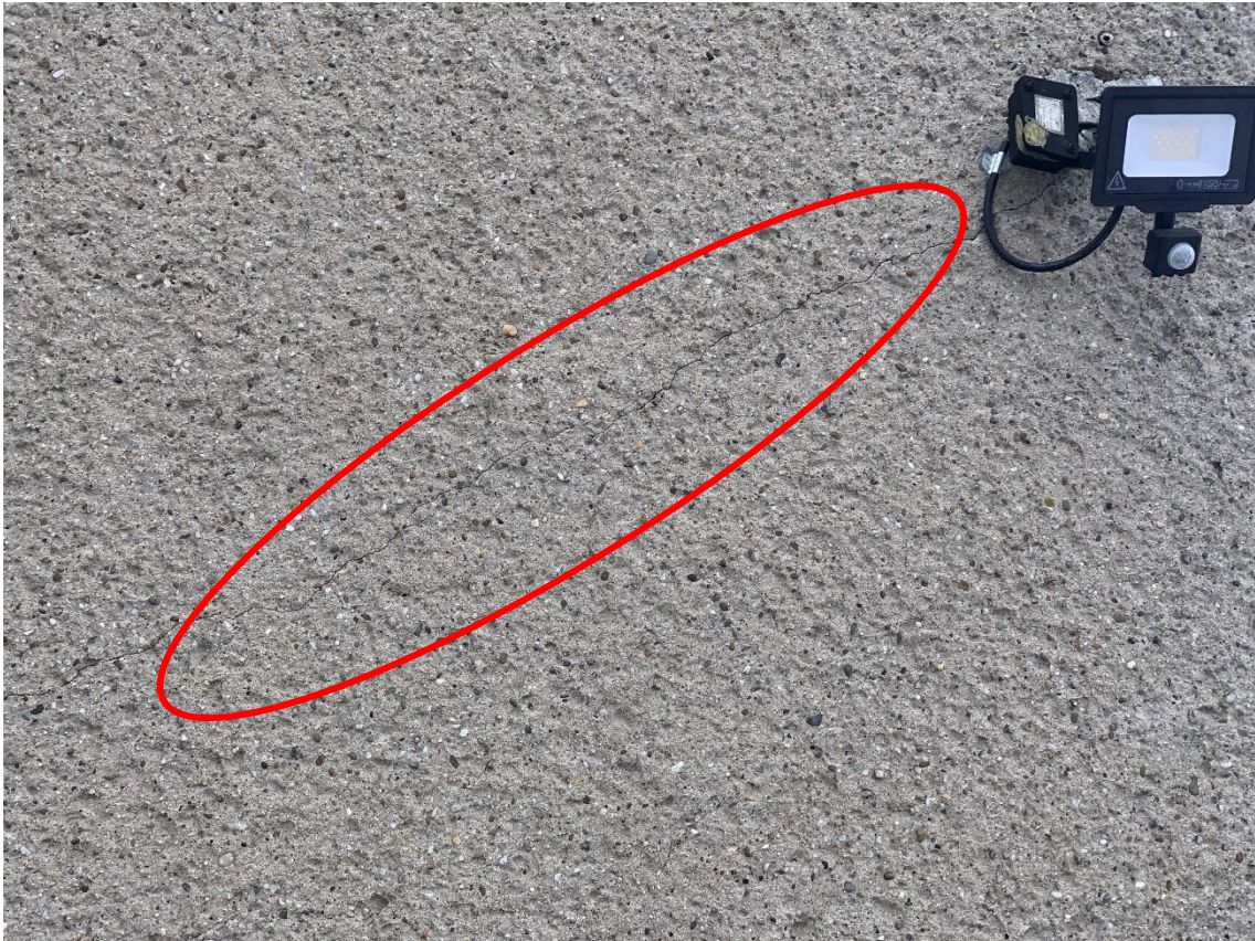
Photograph 3. Visible hairline diagonal crack in the façade plaster ending at a point where a lamp is attached.
