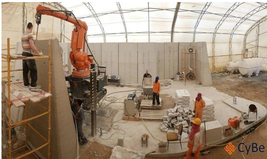
Fig. 4. CyBe Construction CyBe RC 3Dp, CyBe R 3Dp printer [Walasek M., 3d.edu.pl, 2021].
