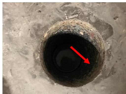
Fig. 2.6. The red arrow indicates water between the floor and the foundation slab.
