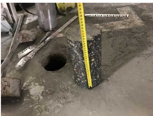
Fig. 2.5. Measuring the thickness of the borehole in the underground garage foundation slab: 27.7 cm.
