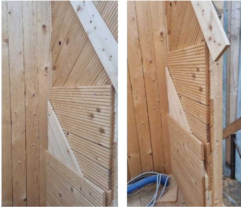
Fig. 23, 24. The method of laying the layers of the external wall (own photos).
