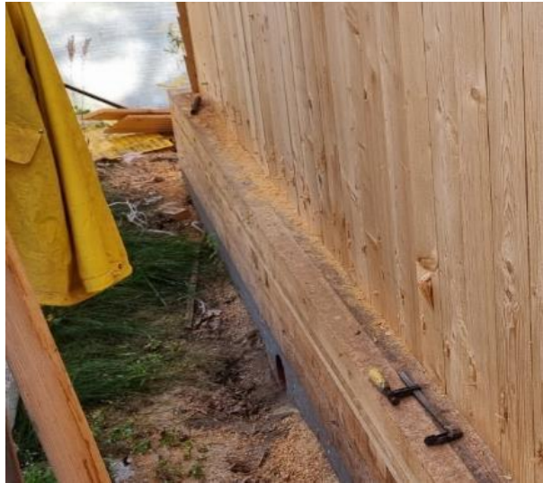
Fig. 9. Ventilation hole (own photos).
