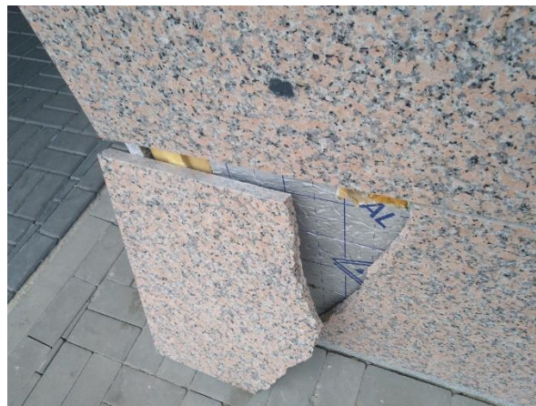
Fig. 7. Result of the impact resistance test of the ventilated façade: the façade system cannot be used in areas accessible to people (Author's photo)
