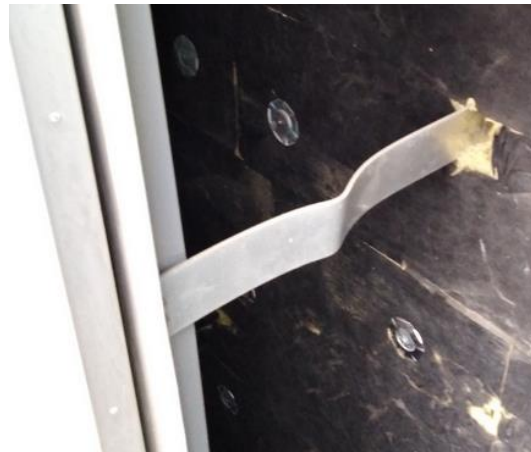
Fig. 6. Damage to the ventilated façade grid (Author's photo)
