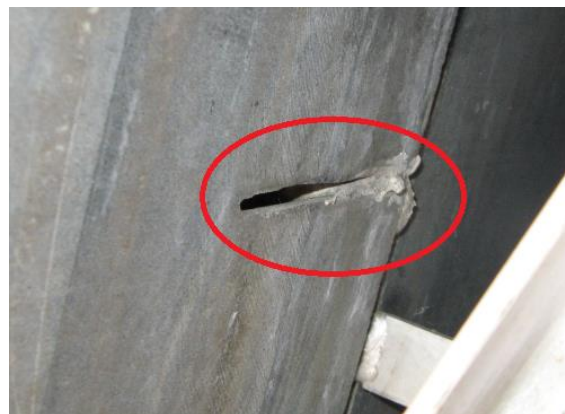
Fig. 5. Damage to "grate - elevation" connections (Author's photo)
