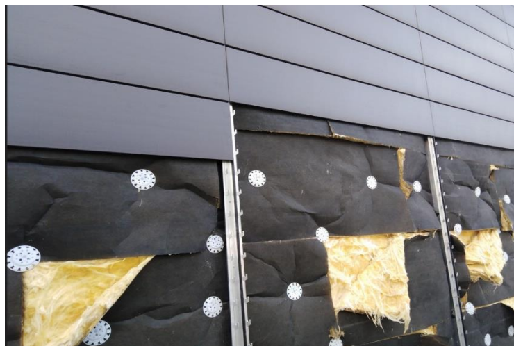
Fig. 4. Expansion of mineral wool leading to disappearance of ventilated space (Author's photo)
