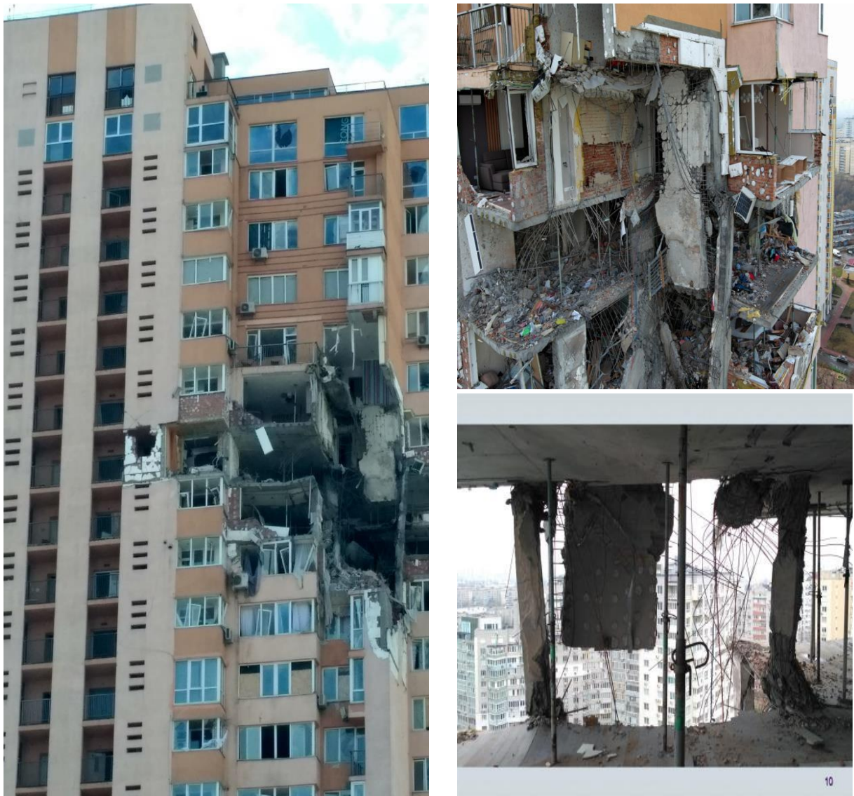
Fig. 3. View of the facade and destruction of structures after a rocket explosion
