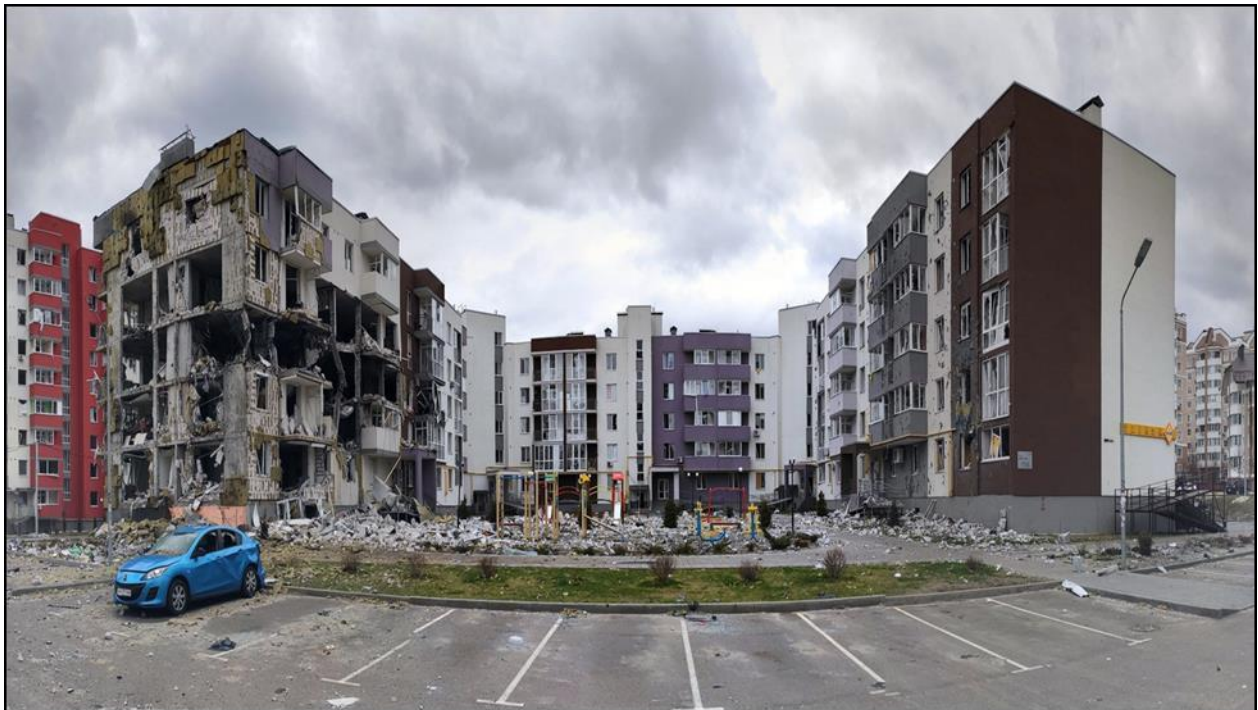
Fig. 2. View of a residential building damaged due to an aerial bomb explosion
