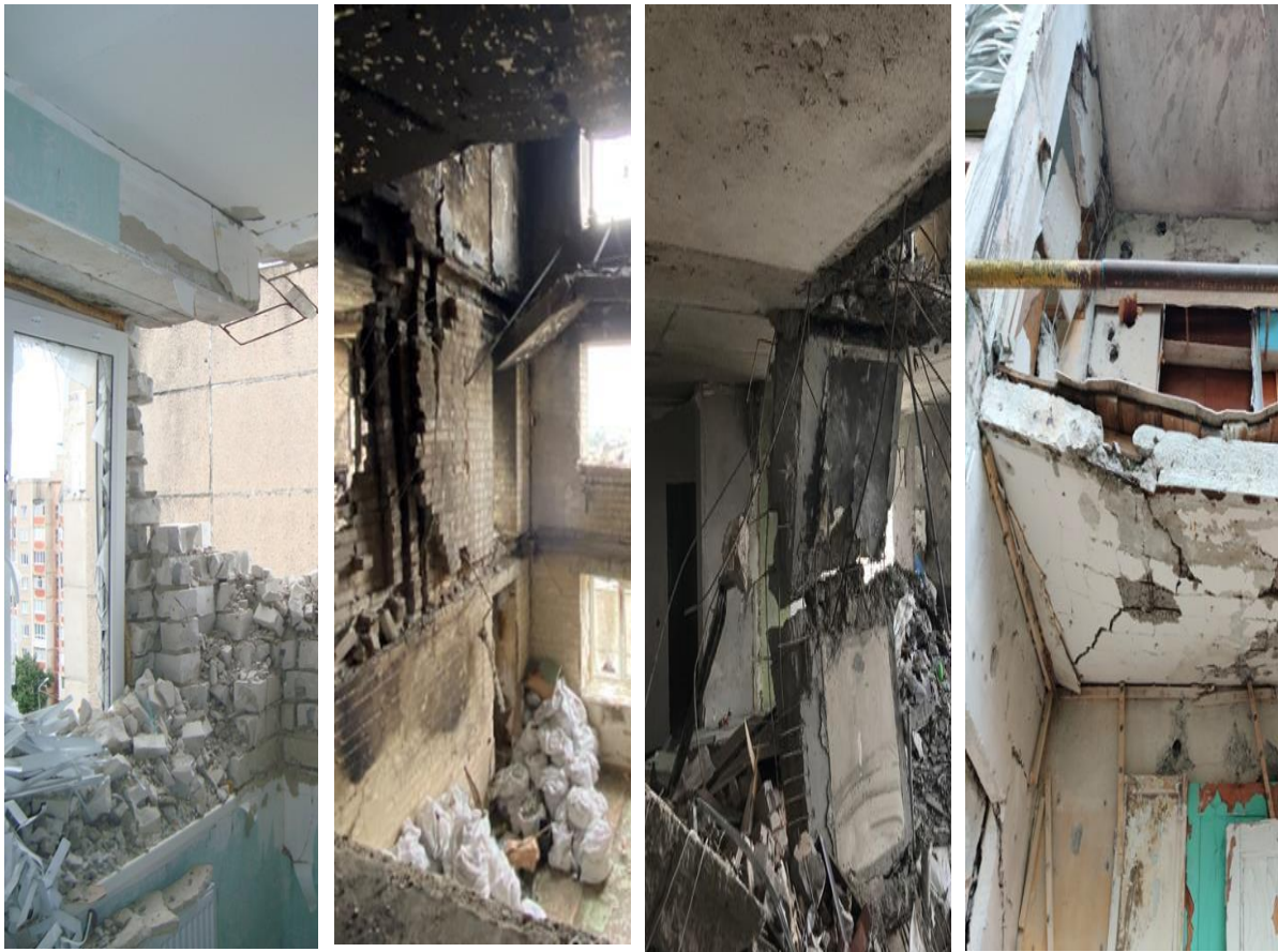
Fig. 6. Consequences of artillery shell explosions in residential buildings
