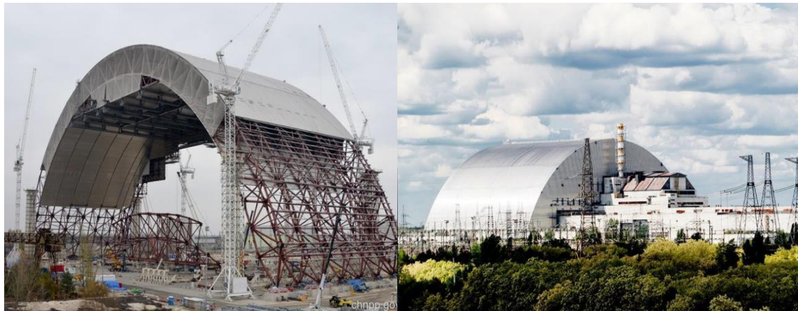
Fig. 9. Construction of the Shelter Facility in the "safe" area of the construction site and general view of the Shelter Facility after construction operations were completed
