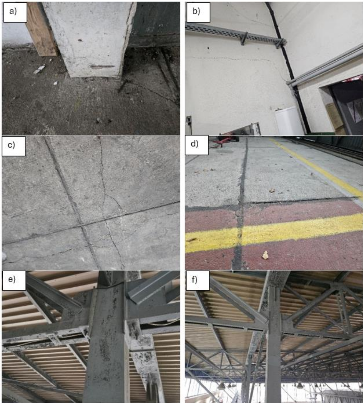
Fig. 2. The condition of the facility: a) damage of the column of supporting structure, b) wall cracks, c, d) condition of the hangar floor, e, f) condition of the steel roof structure.
